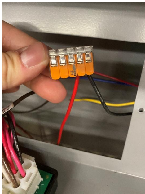
Figure 8: T3 wire connection
